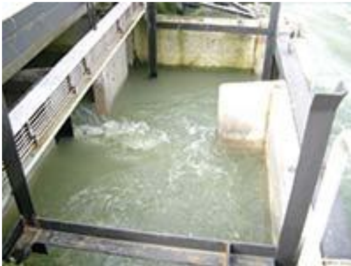
Vertical Slot Fish way in Goolwa Barrage
