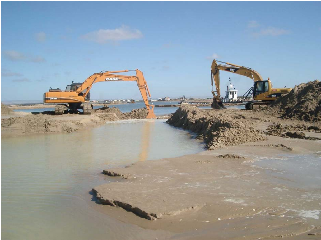
Figure 8. Dredging operations undertaken during 2002/03 to maintain an opening at the Murray Mouth. (Photo: Brenton Erdmann)
